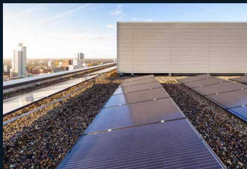
Landmark rooftop solar panels
